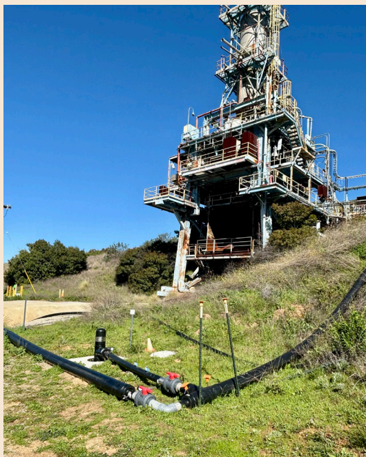
The enhanced in situ bioremediation system in the Alfa Test Area, shown in part above, is one of the treatment technologies in NASA's approved Phase 1 groundwater remedy.
