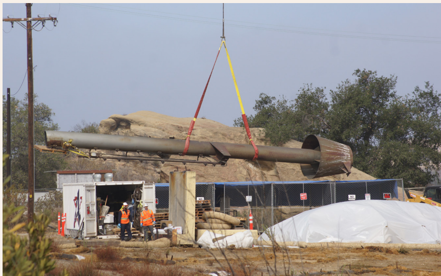
Demolition crews remove one of the three flare stacks, also referred to as “tiki torches” from the top of Bravo Test Stand 2. NASA is donating these flare stacks to the Air Force Flight Test Museum at Edwards Air Force Base.
