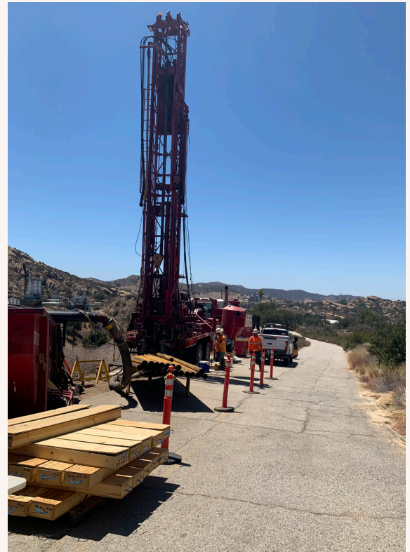
A drilling rig drills one of three injection wells for the EISB pilot studies in the Alfa Test Area at SSFL.
