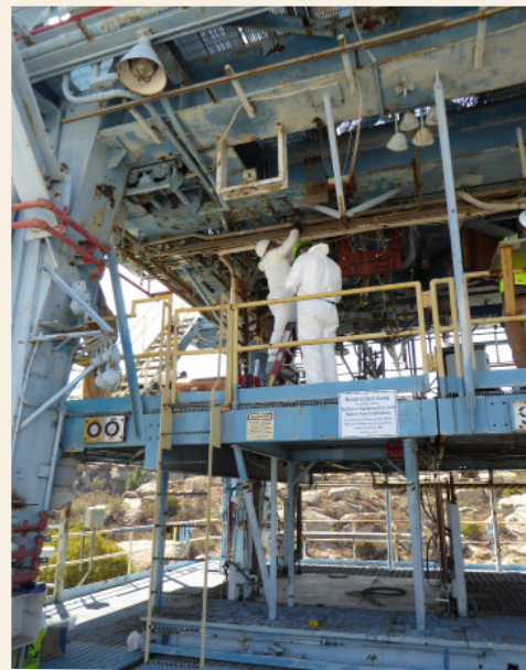
Environmental technicians carefully extract fluids from pipelines at one of the Alfa Test Stands.
