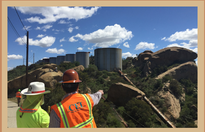
Demolition crew members survey obsolete tanks and pipeline in the Skyline Area scheduled for demolition in Phase 2.
