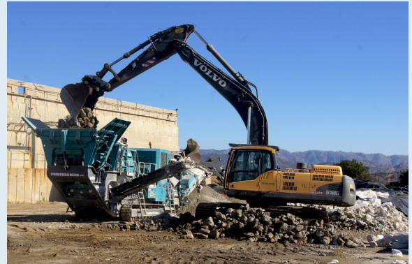
Demolition began in the Service Area in early 2015 and is expected to be completed at the end of 2018.
