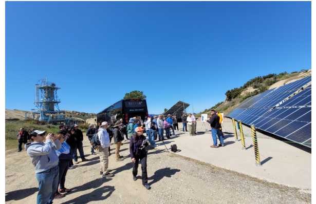
NASA SSFL Project Director Peter Zorba discusses the BVE system with community members during DTSC's Groundwater U site tour in April.
