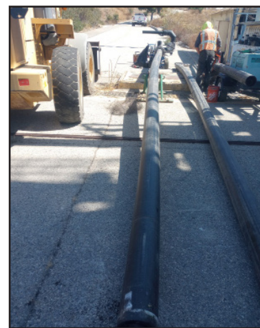
Workers prepare the high-density polyethylene pipeline (HDPE) for the Bedrock Vapor Extraction pilot study system in the Alfa Test Area.
