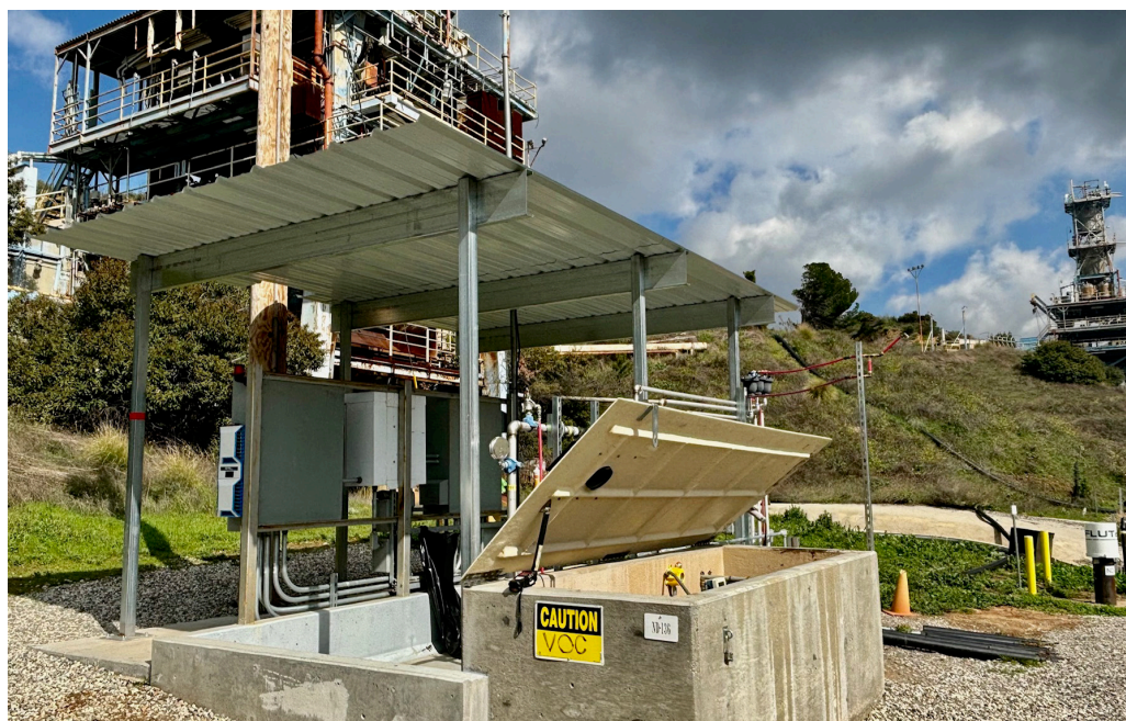
NASA constructed an EISB treatment system for a groundwater pilot study near the spillway of Alfa Test Stand 1.
